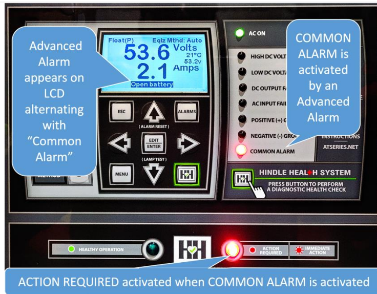
Figure 5 – Advanced Alarm That Triggers the Common Alarm
