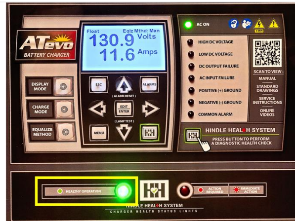
Figure 2A – Status LED for Healthy Operation
